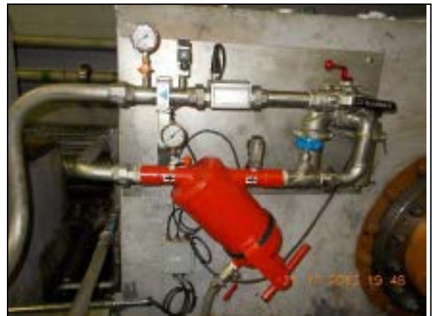
Figure 6 - Water Filtration System
