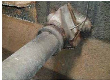
Peak Cap bearing, shaft and grease line
