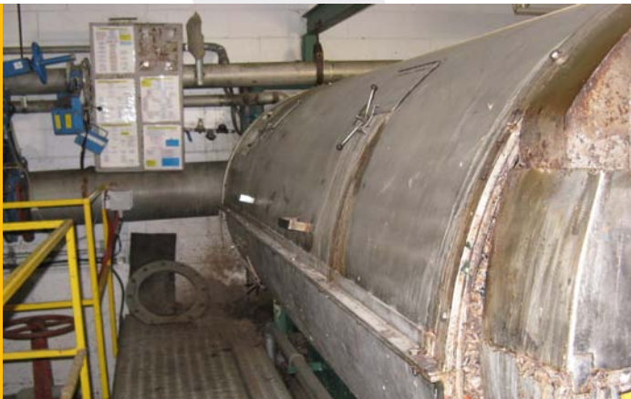
SXL bearings installed in trammel
