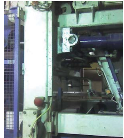
Grease free Thordon SXL installed in press for paving stone manufacturing
