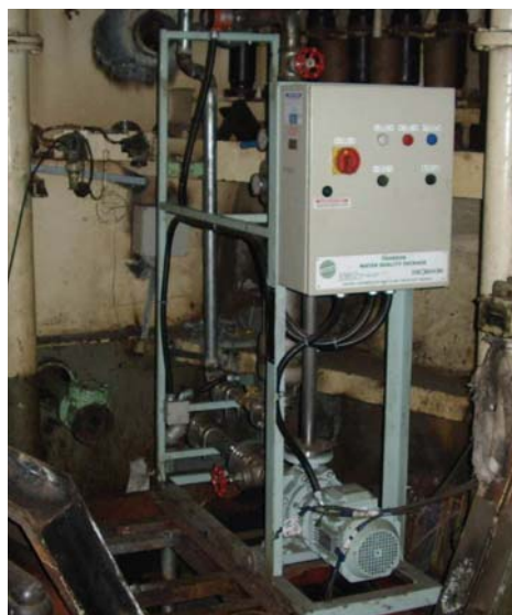
Thordon Water Quality Package installed on CSL Acadian
