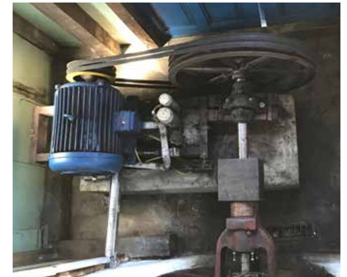
No. 3 Turbine before refurbishment efforts began
