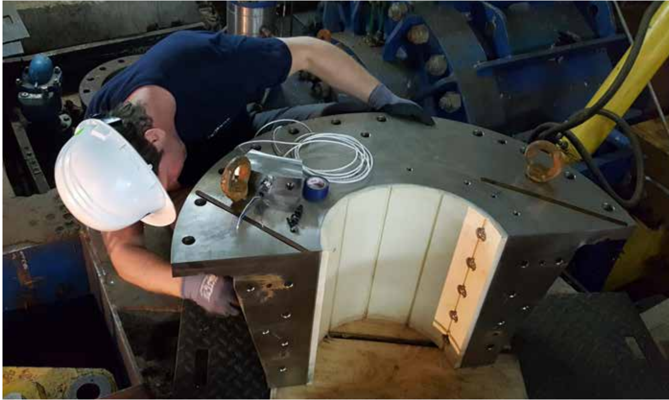
A member of the Global Service & Support team installing an SXL guide bearing in a split stainless-steel housing
