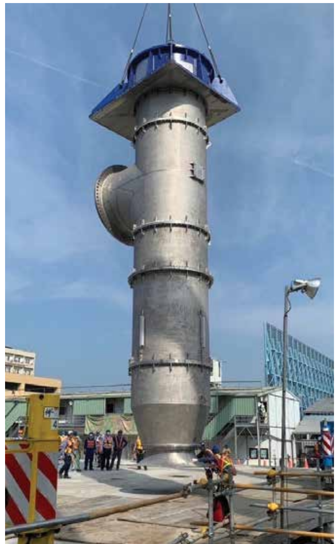
One of the pumps fitted with Thordon’s non-metallic pump bearings ready to be installed.
